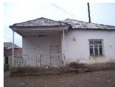
Former building of the barely operating preschool in Margahovit village before Save the Children's intervention: a typical state of many rural preschools in Armenia
